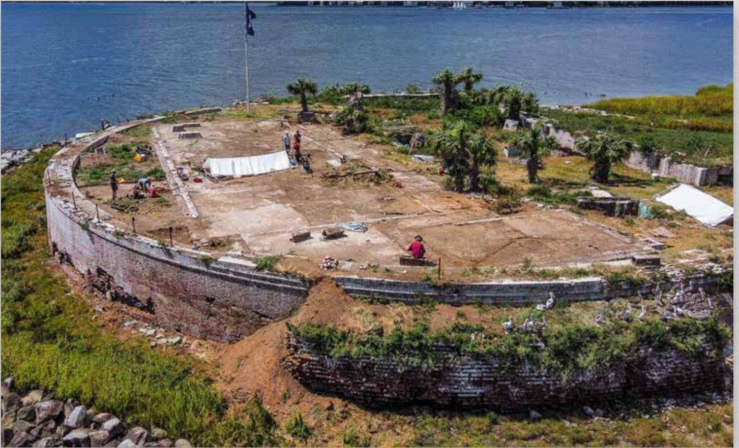
Aerial view of Castle Pinckney after brush and debris removal. (Jason Parker)
